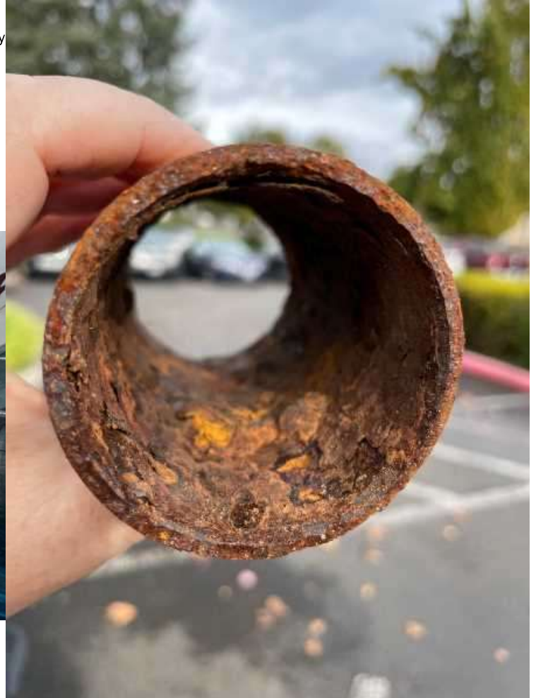
COURTESY PHOTO: CITY OF OC - Oregon City replaced a corroded and undersized pipe this year on Latourette Street.
