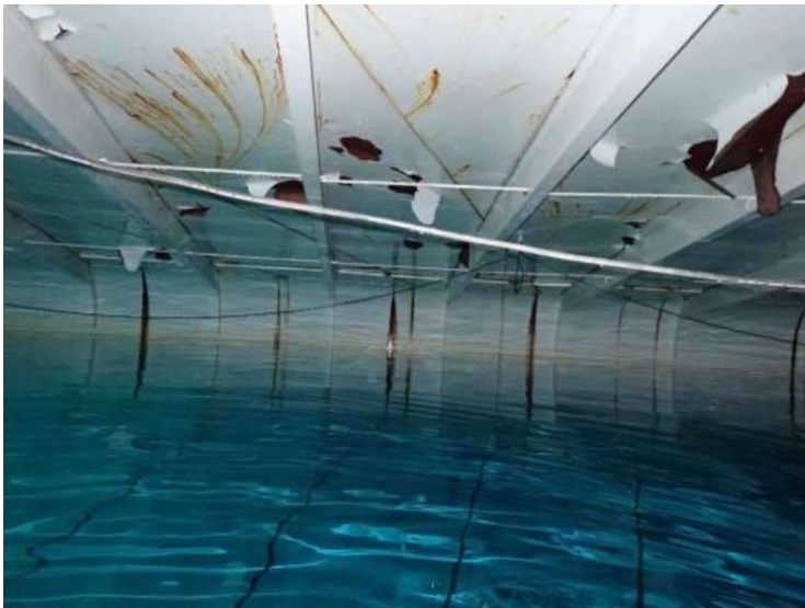
COURTESY PHOTO: CITY OF OC - Paint is peeling from the ceiling of the Henrici Reservoir in Oregon City.
