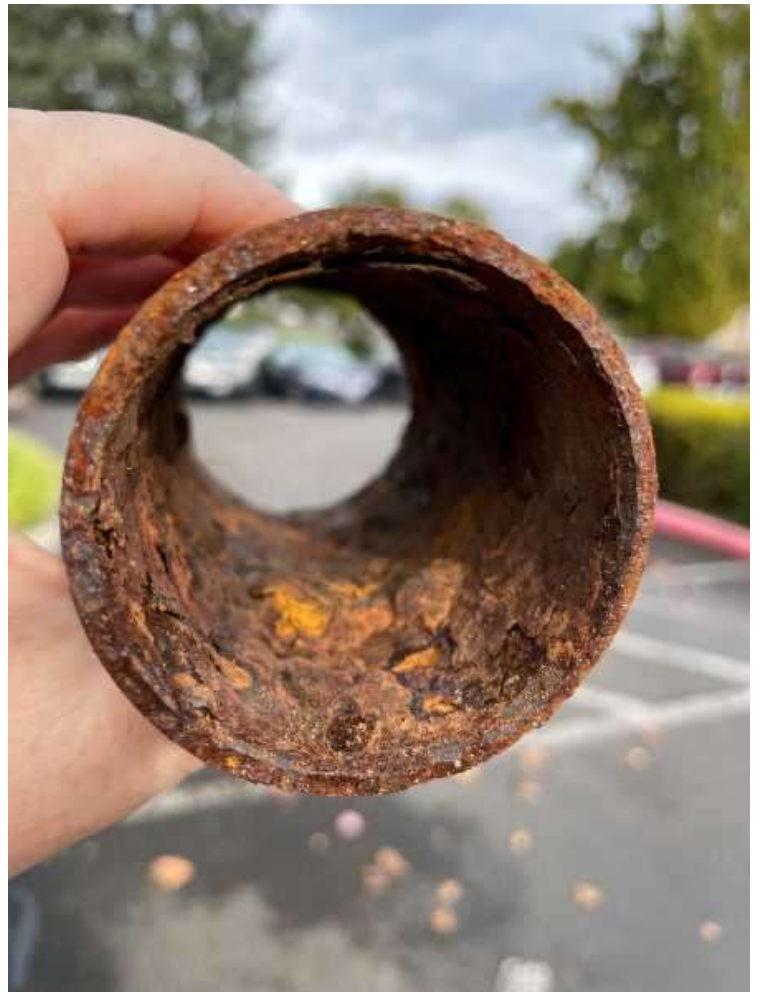
COURTESY PHOTO: CITY OF OC - Oregon City replaced a corroded and undersize pipe this year on Latourette Street.
