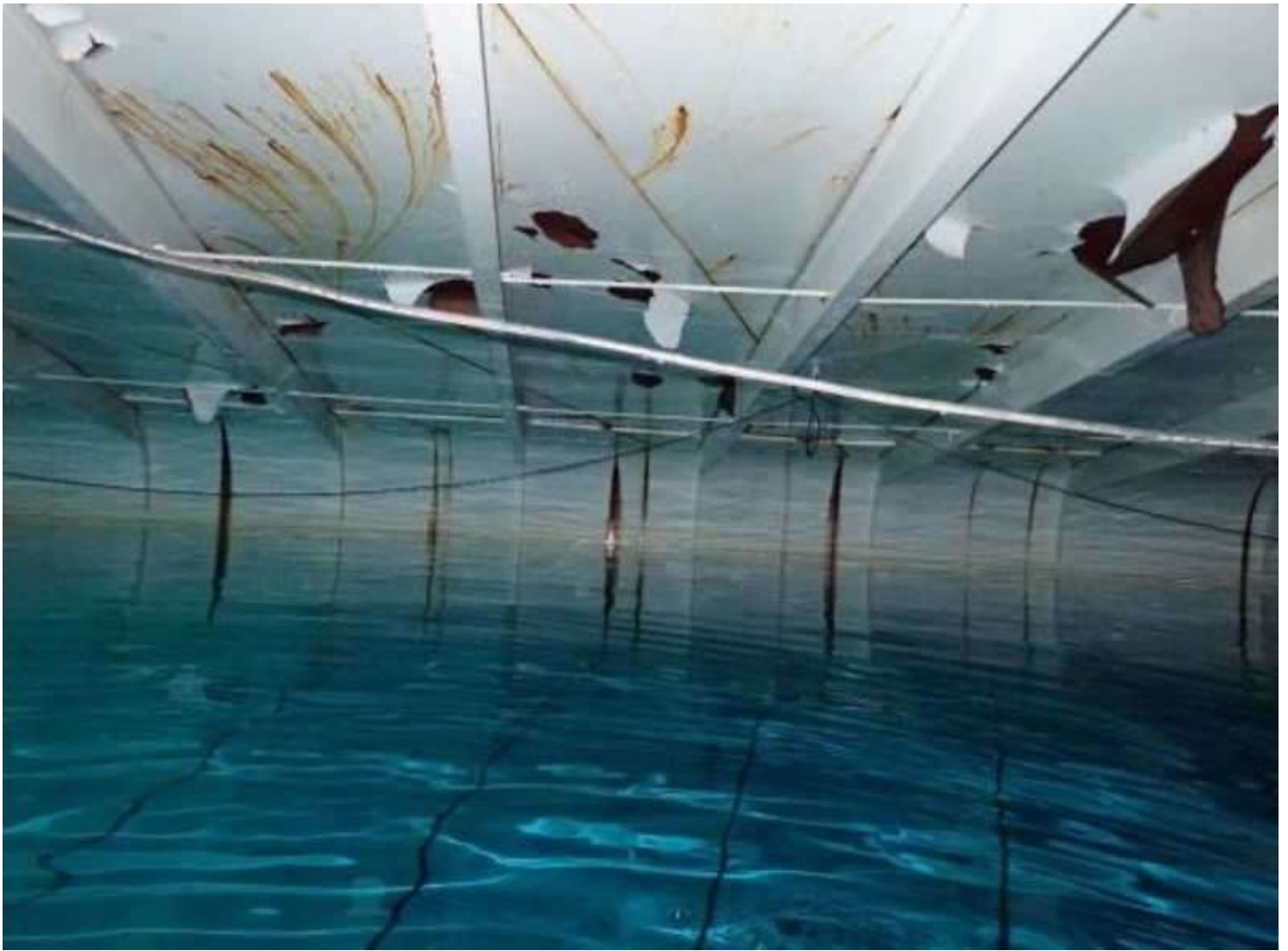
COURTESY PHOTO: CITY OF OC - Paint is peeling from the ceiling of the Henrici Reservoir in Oregon City.
